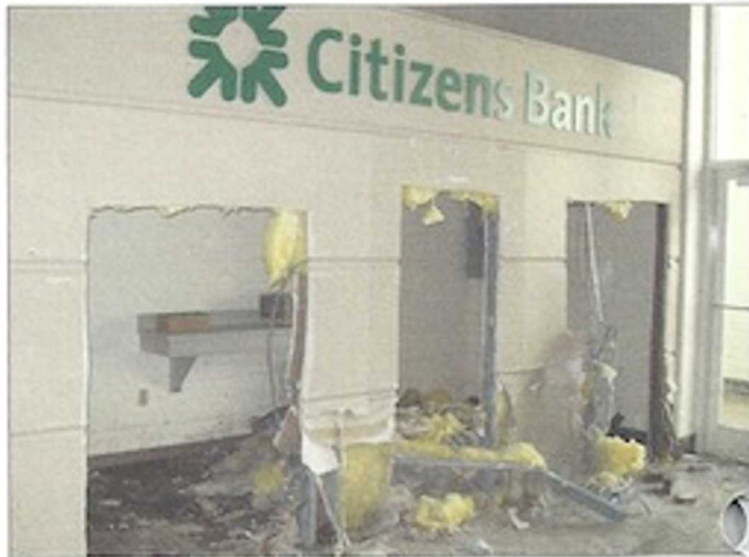
Citizens Bank's ATMs and night deposit vaults at Warwick Mall had to be removed, after sitting in two feet of water for days.
