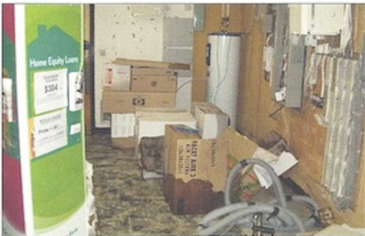
Basement flooding impacted several branches, including Mineral Spring Avenue in North Providence.
